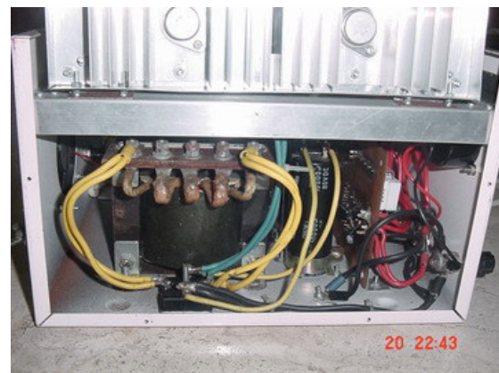
Tampak samping Trafo & Diode Bridge
